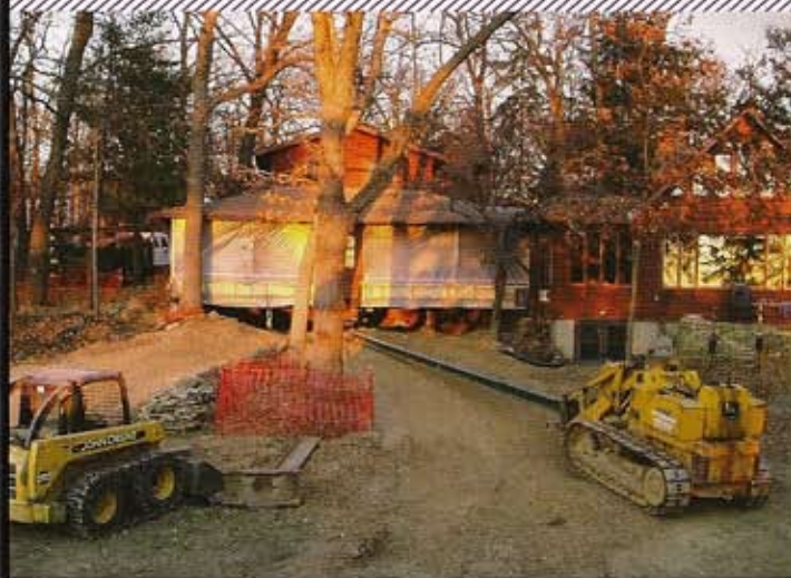
Cementing the connection between historic preservation and sustainability, TDS Custom Construction dug out the soil from around this Madison home without damaging the oaks surrounding it.
